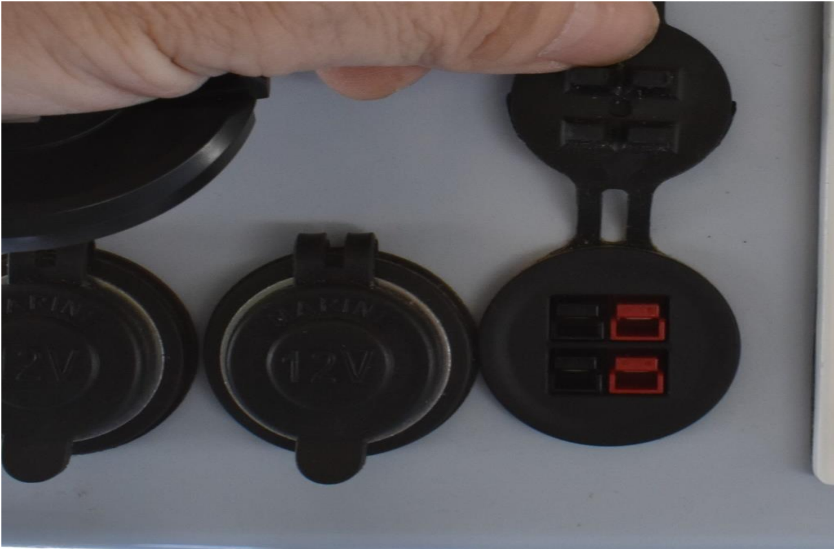
Figure 7. 12-Volt Power Outlets and Anderson Powerpole Outlets.
