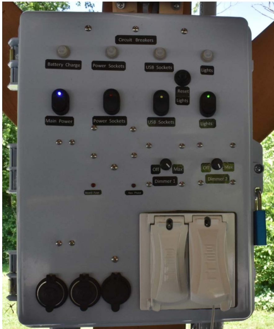
Figure 5. Solar Power Distribution Panel
